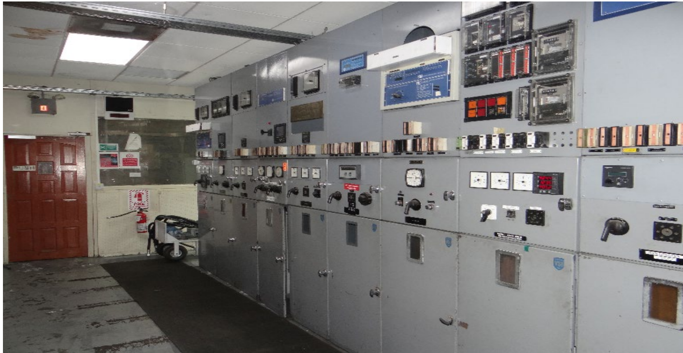
Existing 11 kV switchgear in Fond Colé
