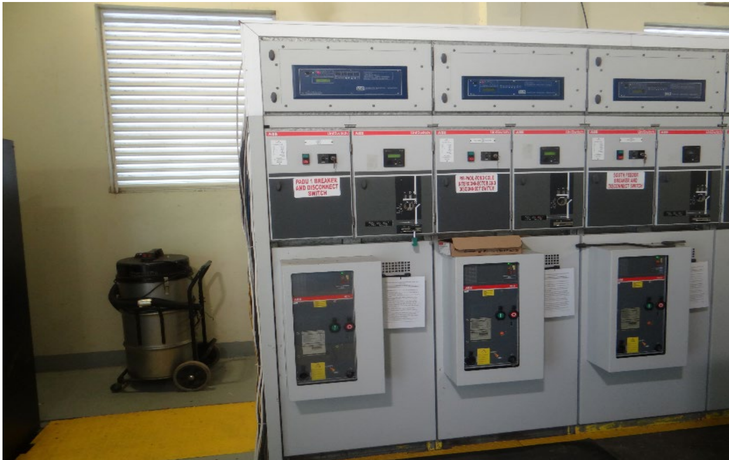
Existing 11 kV switchgear in Padu
