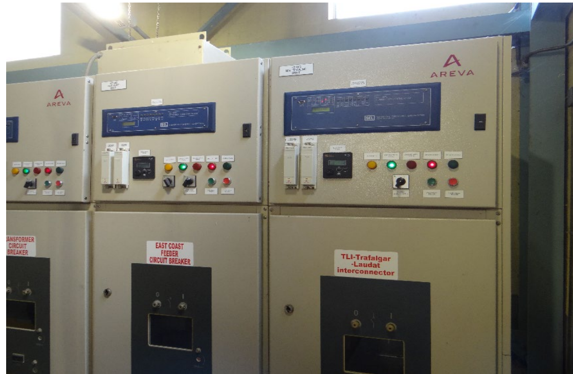
Existing 11kV switchgear in Laudat
